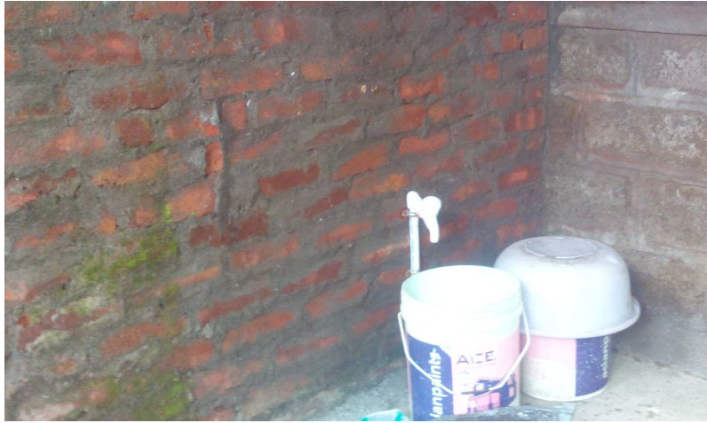
Figure 3 Unplastered bathroom walls, habitat of sand flies
